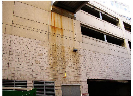
RUST STAIN REMOVAL
